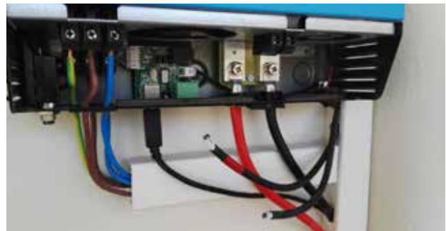
Figure 42: Cable detached from inverter
