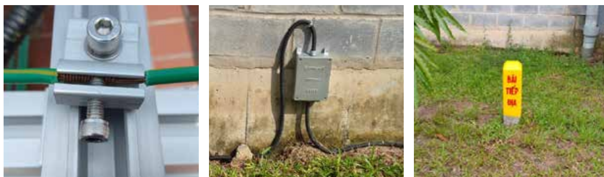
Figure 8: Grounding wire connected to the mounting structure, grounding test box, and grounding field
