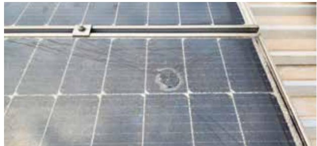
Figure 37: Examples of physical damage on PV panels
