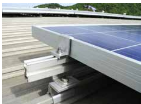
Figure 3: PV panel mounting structures
