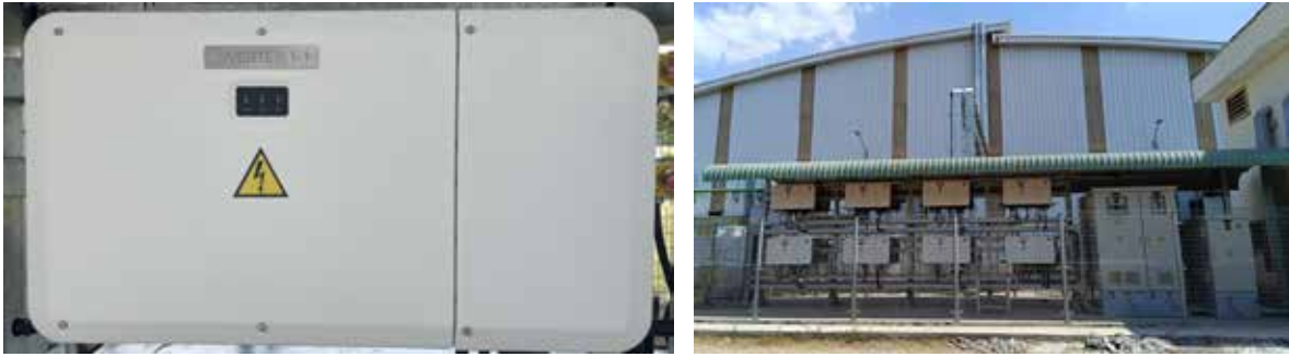
Figure 5: Inverter and inverter placement
