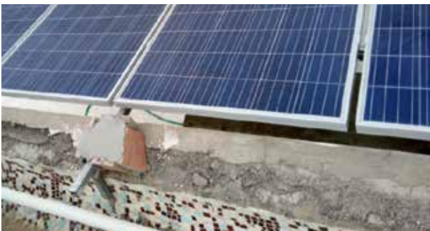
Figure 38: Mounting structures installed inadequately
