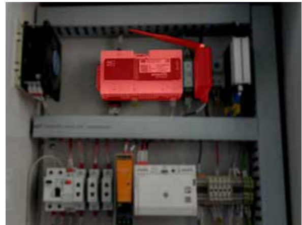
Figure 13: Datalogger (left) and 4G modem (right) installed in the communications cabinet
