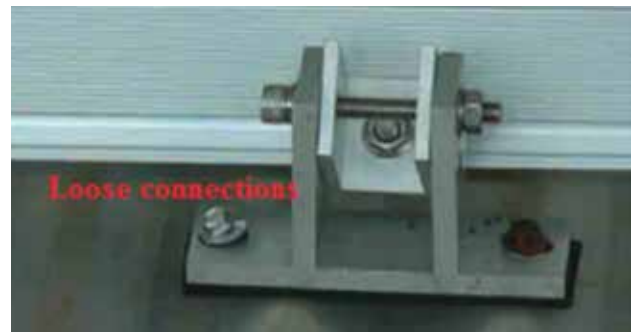
Figure 39: Loose bolts on mounting structures
