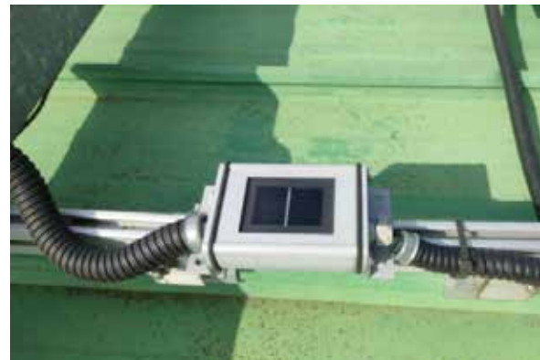
Figure 11: Solar irradiation measurement sensor
