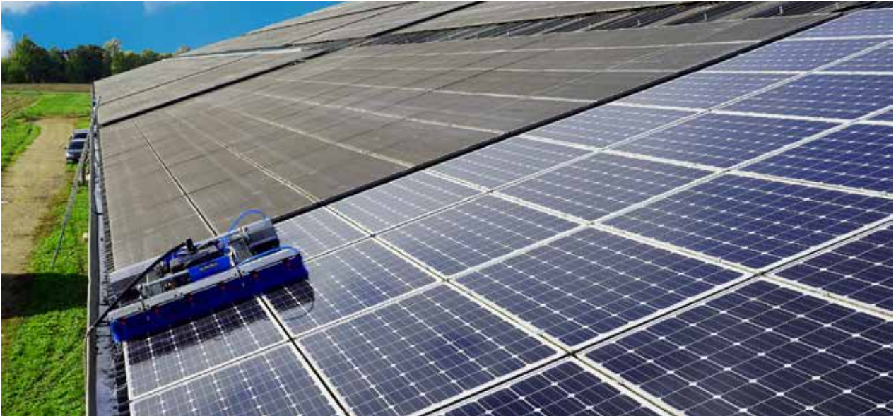
Figure 64: PV panels being cleaned with a biodegradable cleaning chemical 7
