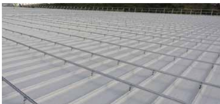
Figure 4: RTS system mounting structures installed on a metal roof
