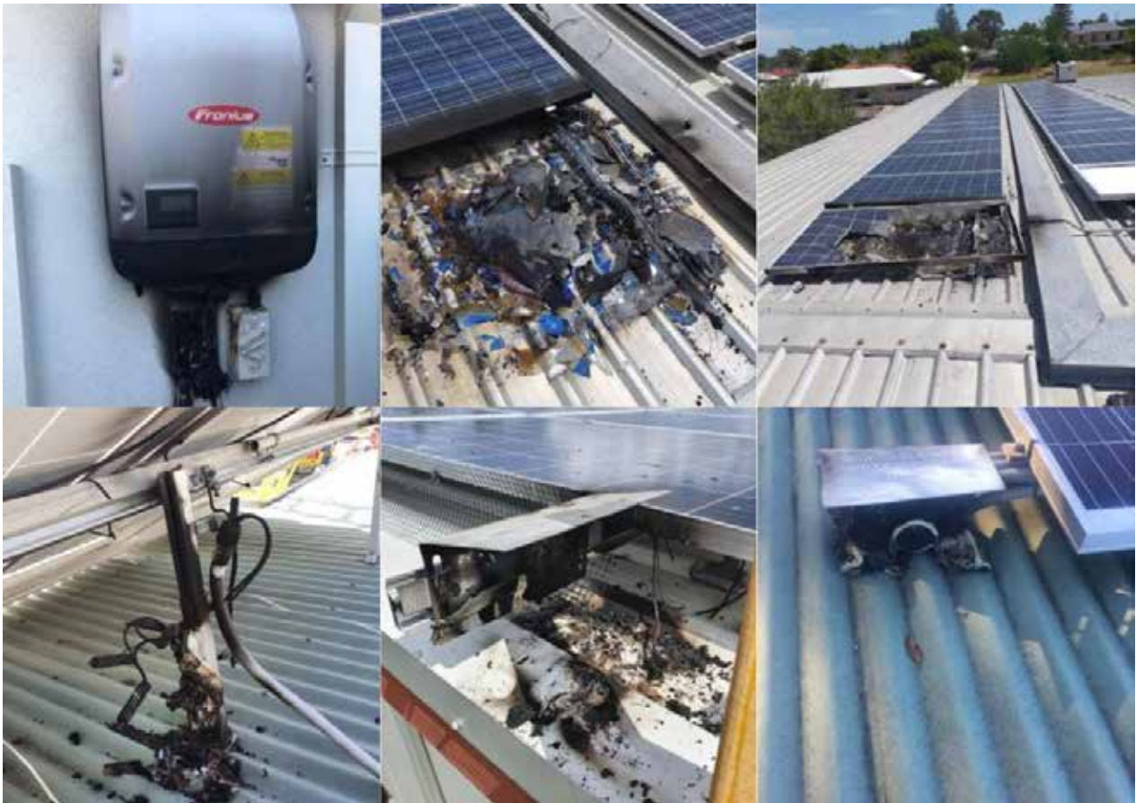
Figure 55: PV panels, inverters and other equipment are burned or exploded
