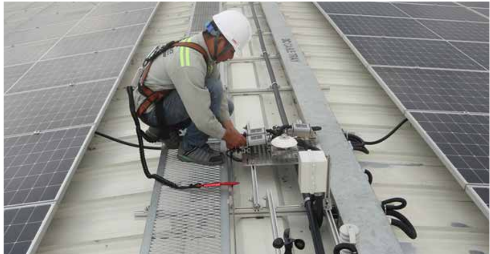
Figure 53: Workers are fully equipped with safety belts when working on a roof
