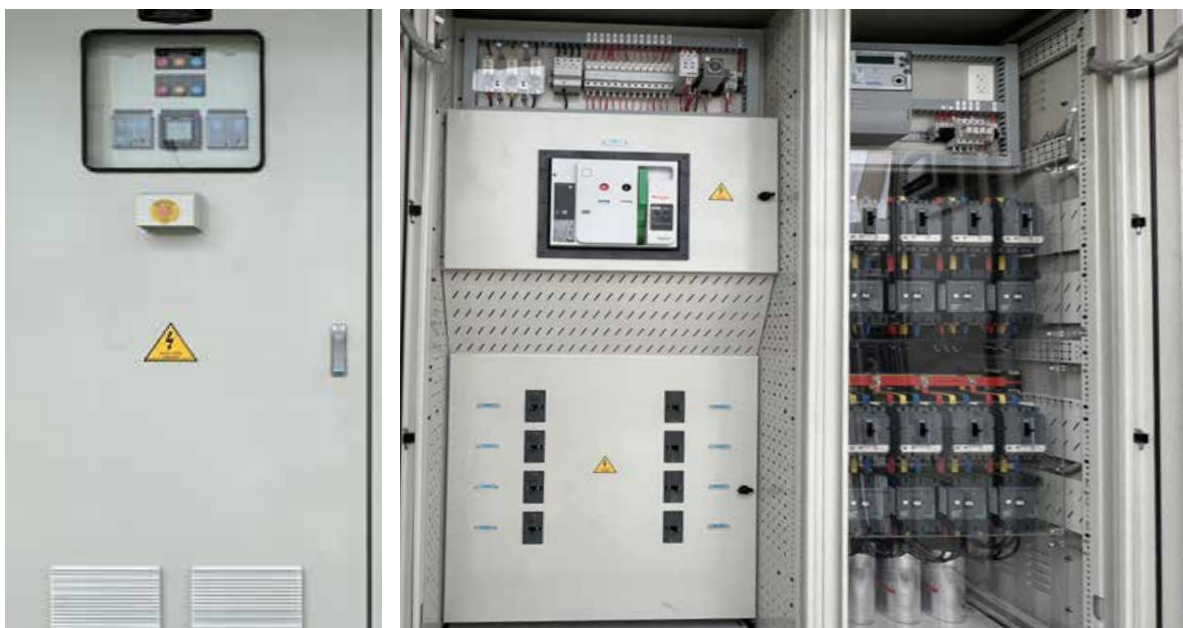
Figure 6: Outside and inside the AC distribution board
