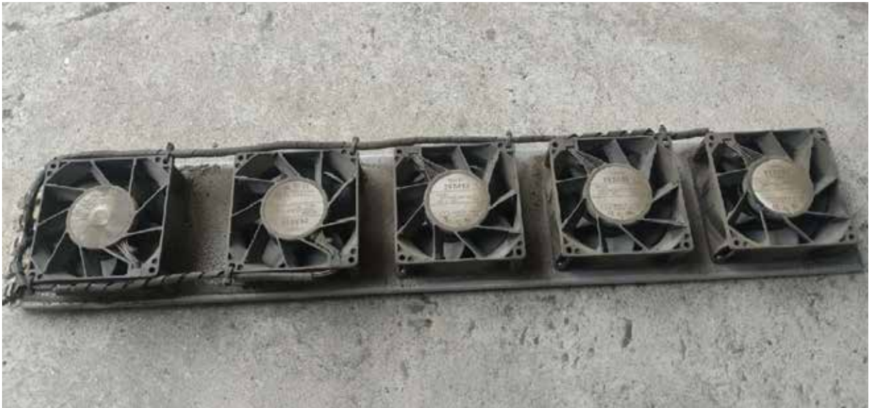
Figure 43: Dust accumulation on inverter
