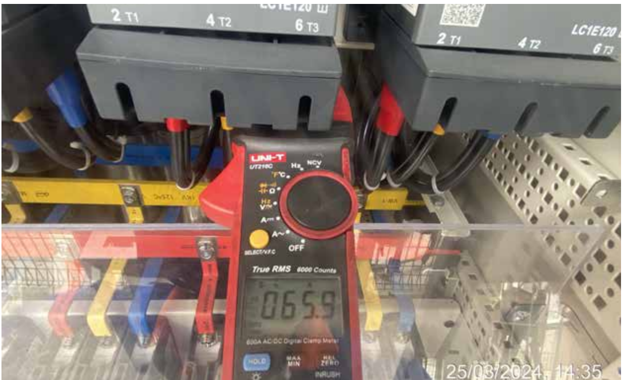
Figure 50: Using a clamp meter to measure current
