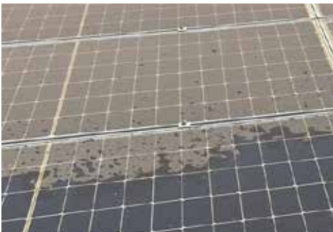
Figure 26: PV panel with dust accumulation
