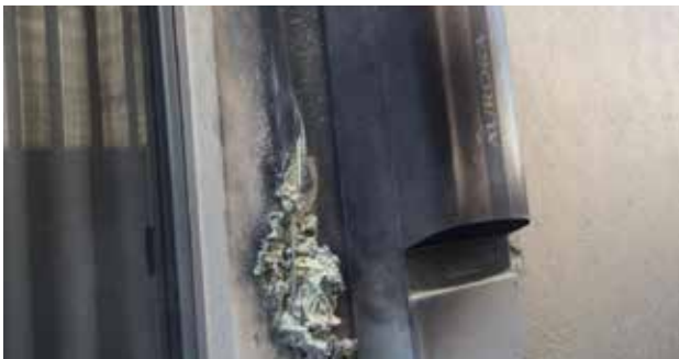
Figure 41: Burnt, damaged inverter
