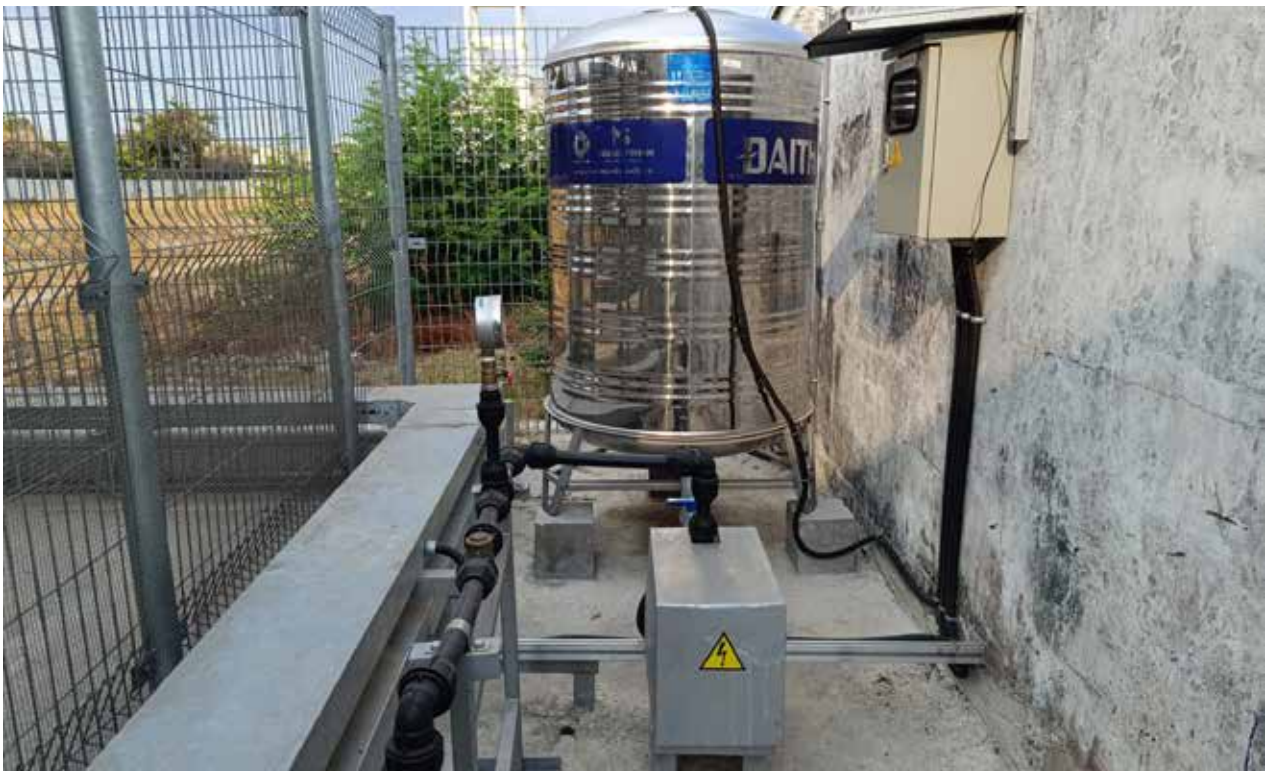
Figure 29: Clean water storage tank and pump for cleaning PV panels
